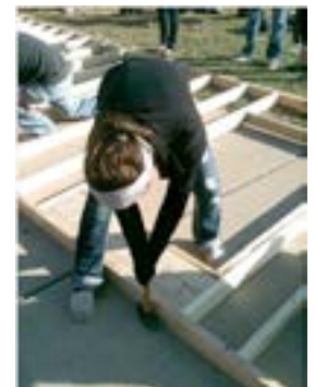
Members of GEC partnered with Habitat for Humanity to help build a house for a local Springfield family.
